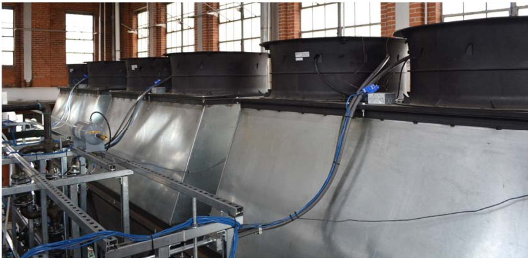
Figure 4-29. Cooling cycle condenser fans on top of the sheet metal reductions
