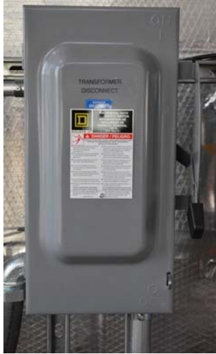
Figure 4-67. Transformer disconnect switch.
