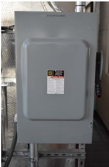
Figure 4-69. Air heater disconnect switch.
