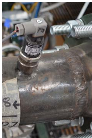
Figure 4-71. Absolute pressure transducer installed in pipe.
