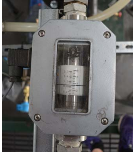
Figure 4-79. Bearing drain line volumetric flow meter.
