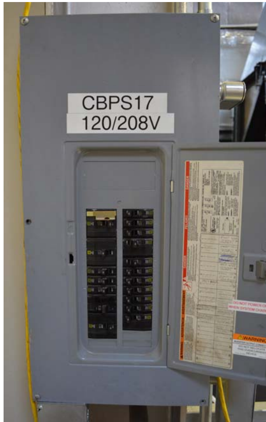
Figure 4-70. 120VAC powerhouse distribution panel.
