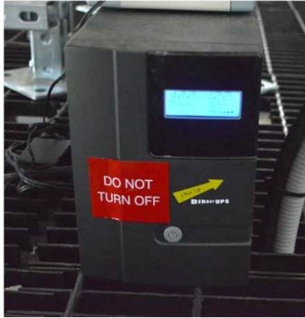
Figure 4-14. The UPS maintains power to EMB systems in a power loss scenario.
