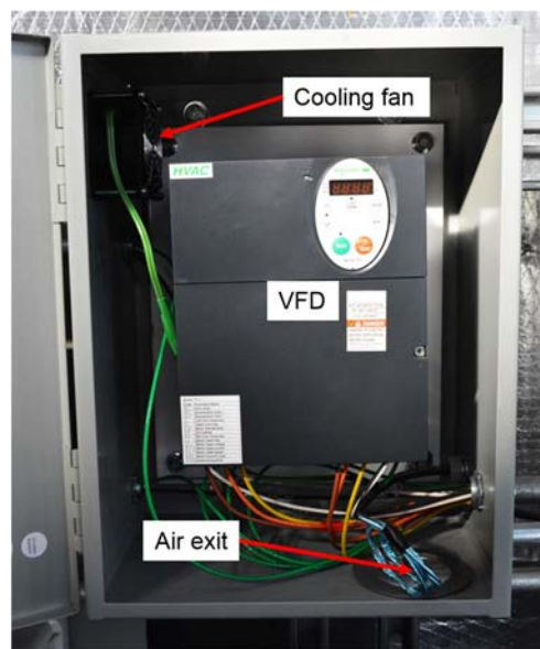
Figure 4-37. Tunnel circulation fan variable frequency drive.
