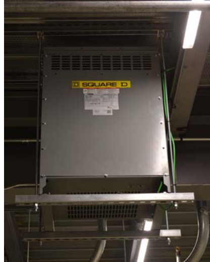
Figure 4-68. Transformer located beneath the mezzanine.
