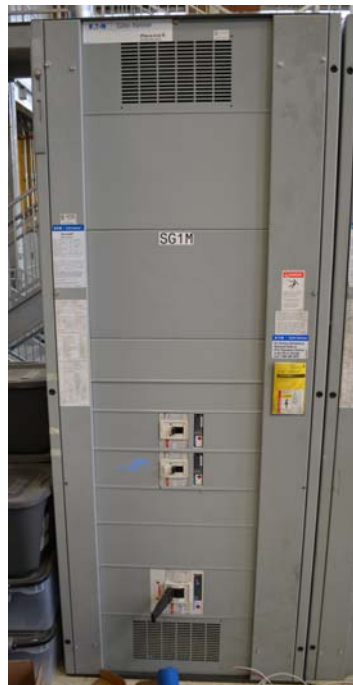
Figure 4-65. Switchboard for the TCCS.
