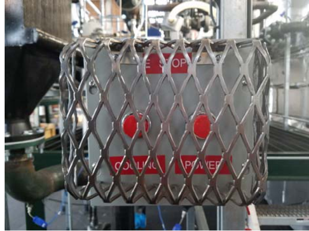
Figure 4-15. EMB buttons located on the mezzanine. An identical box is located in the control room.
